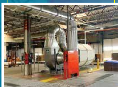
Dust collector & air filtration
