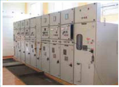
Electric Control Room
